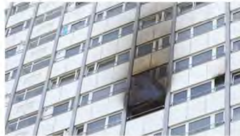
Smoke damage at Queensdale Crescent
