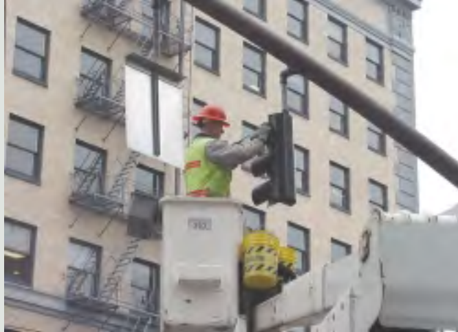
A City-bired contractor installs one of more than 13,000 LED lamps during the fall of 2001.
