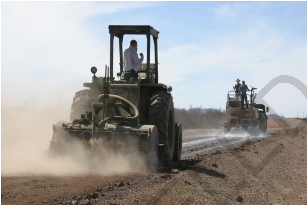
Figure 5-2 Applying Product with Hydroseeder and Mixing into Road Surface with Rotary Mixer
