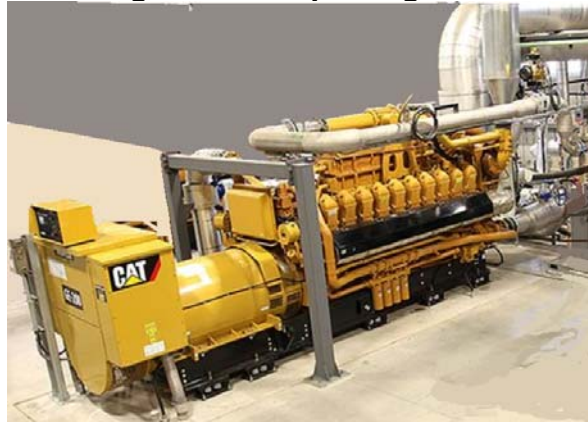
Reciprocating engine CHP system
