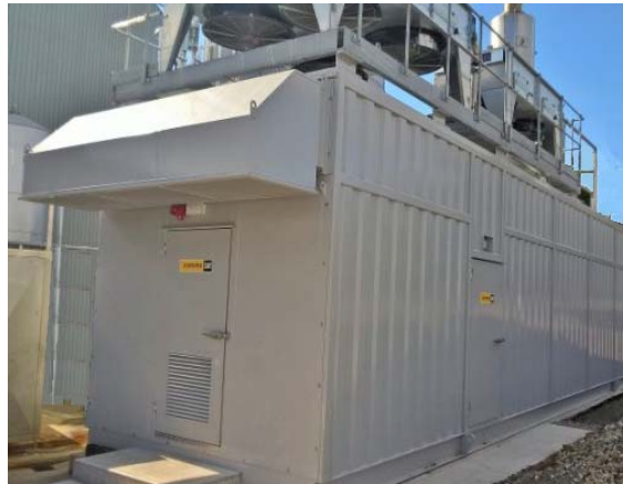
Small gas turbine packaged CHP
