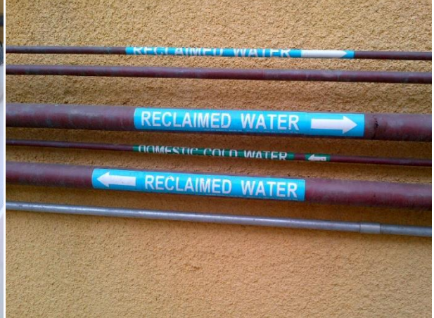
Figure 2. Purple Pipe for building reuse at a DoD training barracks. (Source: USACE, ERDC-CERL)
