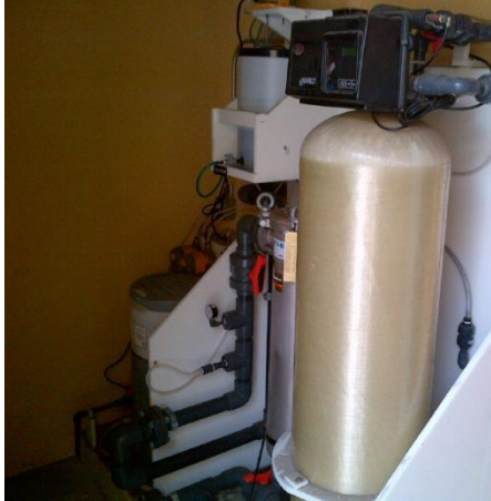
Figure 1. Gray water treatment system in an out-building at a DoD training barracks. (Source: USACE, ERDC-CERL)
