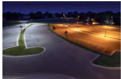
LED parking lot lights (left) compared to HPS lights (right) show different color appearance and more uniformed light distribution.
