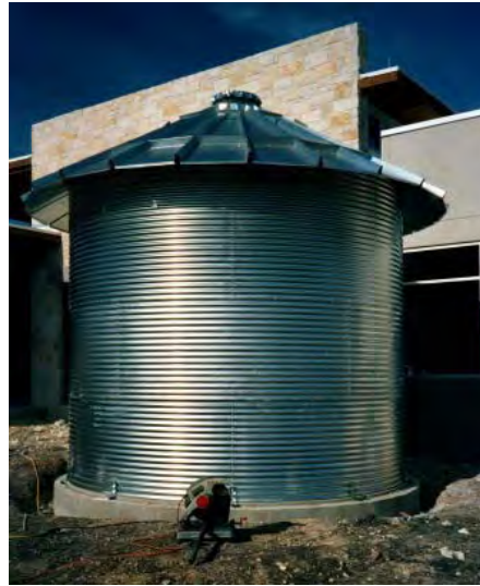
Figure A9. Galvanized sheet metal tank (source: TWDB 2005).
