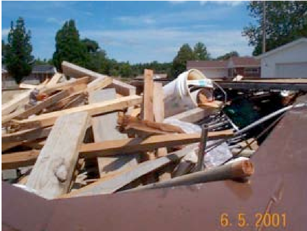
Figure 3-8. Accumulated waste, Fort Campbell remodeling site.
