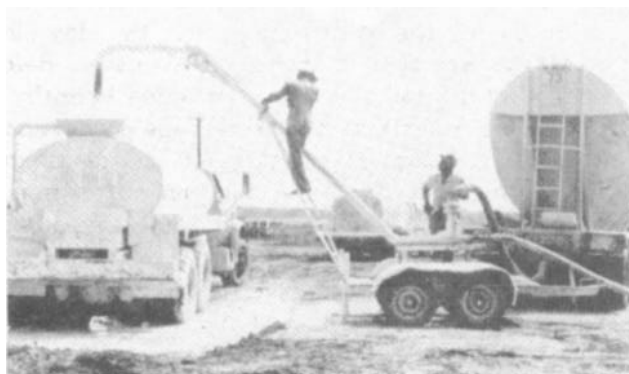
Figure 4-30. Jet slurry mixing plant.
