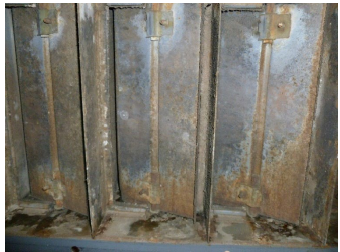
Rusty damper blades still work in 40-year-old unit.
