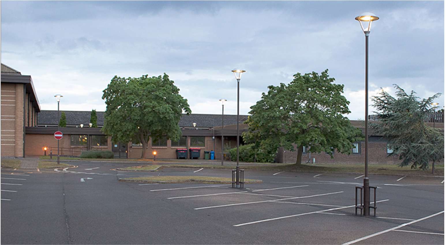
Standard Lighting at Parking Lot
