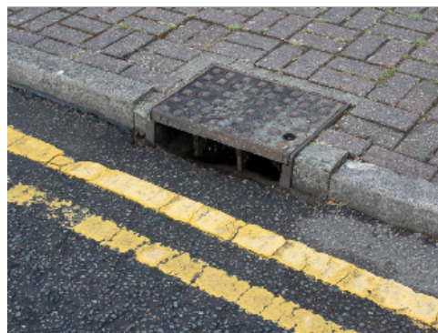
Storm Drain at Street
