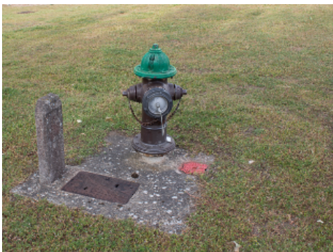
Standard Fire Hydrant
