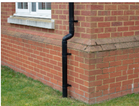
Downspout to Underground Drainage
