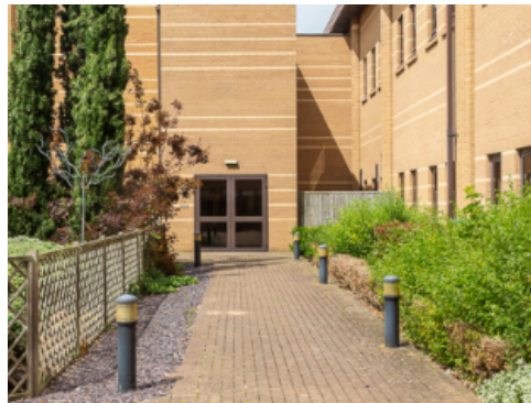
Bollard Lights at Hospital
