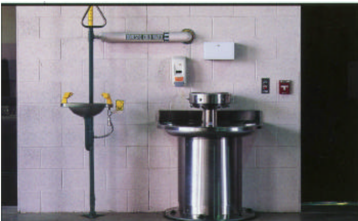
Emergency shower/ eyewash and gang foot-activated hand washing stations should be in open, easily accessible areas
