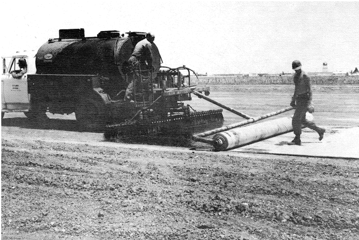
Figure 3-2. Rolling frame for placing polypropylene fabric over the first coat of asphalt emulsion.
