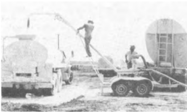
Figure 4-30. Jet slurry mixing plant.
