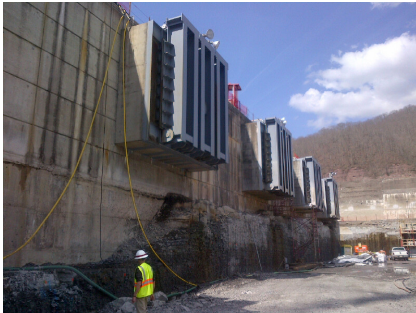
View of the closure gates on the existing penstocks.
