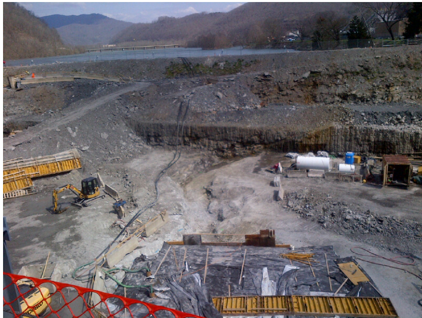
View of the stilling basin excavation. Work in center of picture is a fault that runs upstream to downstream. The fault is being excavated and filled with concrete.
