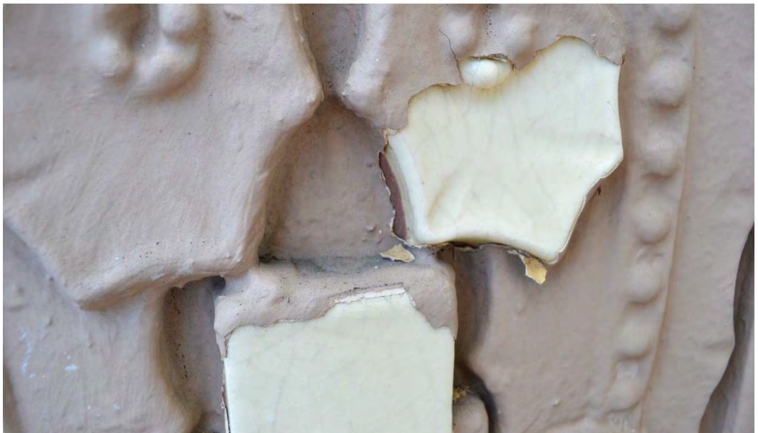
Figure 39. Detail of original ornamental terra-cotta under peeling paint (photo by HHM, 2014).
