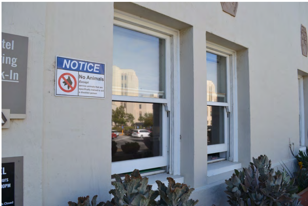
Figure 45. Example of original one-over-one wood-sash windows on Building 9. Historic photographs show that steel casement windows originally were present on Building 9, but the style and construction methods of these windows suggest that they likely date from the 1930s or 1940s. It is unclear whether or not the wood windows were installed during the period of significance (1934–1941), and historic research would be required to determine the exact dates of the windows (photo by HHM, 2014).
