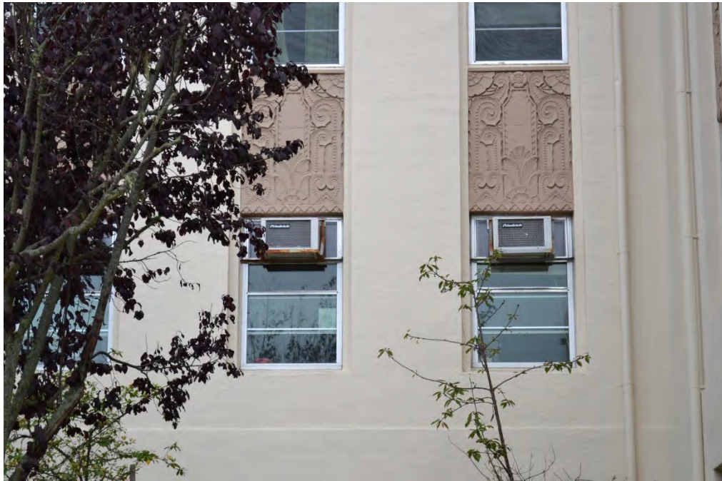
Figure 50. Photo of non-historic window units installed in the non-historic windows at Building 1 (photo by HHM, 2014).
