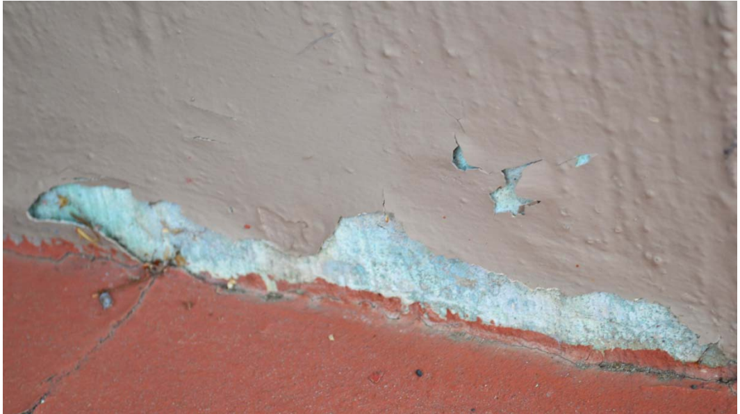
Figure 38. Detail of paint peeling from stucco in a typical exterior entryway (photo by HHM, 2014).
