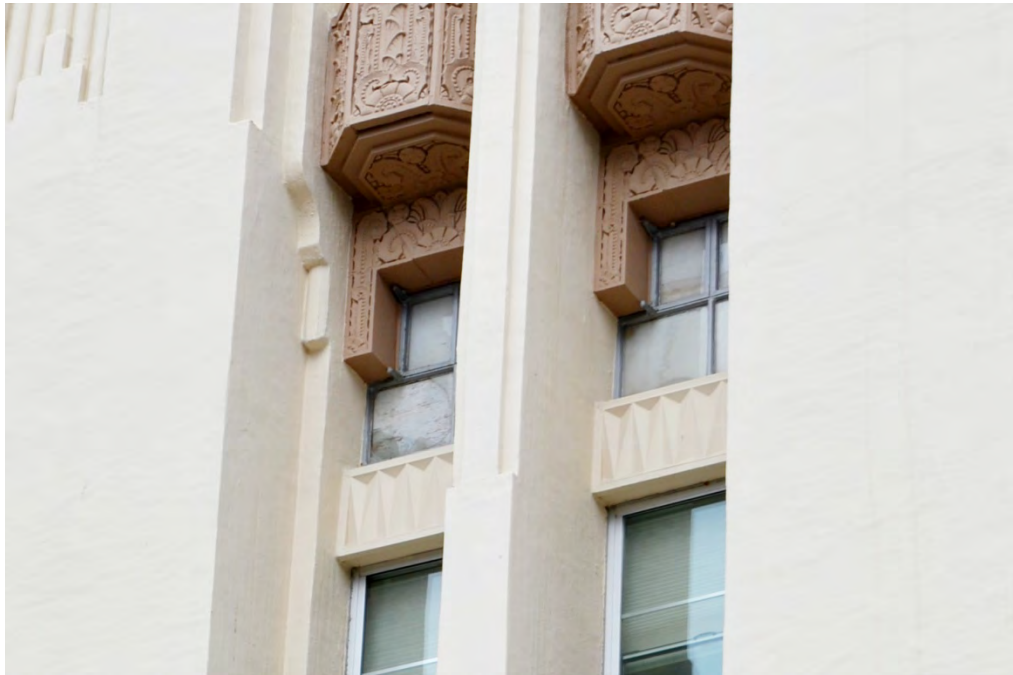
Figure 43. Detail of windows at the tower on Building 1, showing original steel frame windows above newer, non-historic aluminum frame windows (photo by HHM, 2014).
