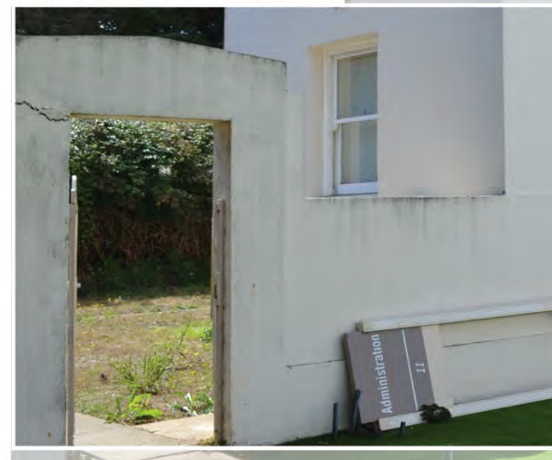
Concrete wing wall and gate opening with stepped pediment and wrought-iron gate
