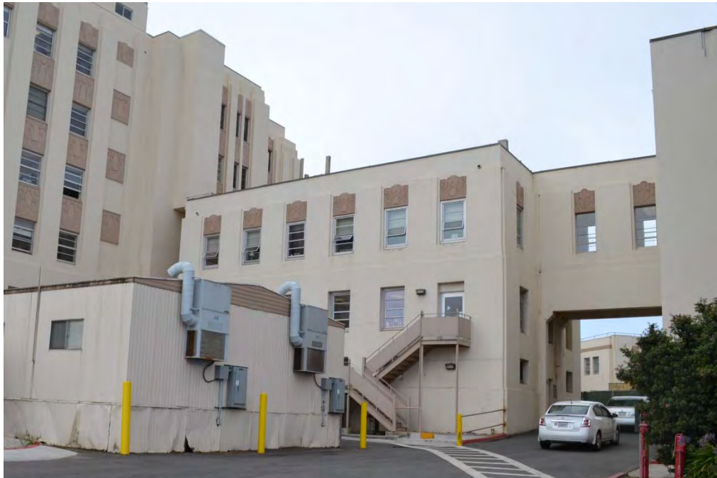
Figure 44. Non-historic aluminum double-hung windows on Building 2 (left) and non-historic aluminum windows on Building 4 (right) (photo by HHM, 2014).
